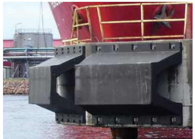
Turning Dolphin | Muuga | Estonia
