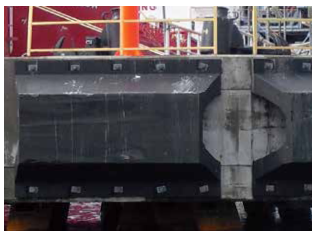
Turning Dolphin | Muuga | Estonia
